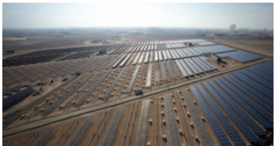
A 10 megawatt photovoltaic power plant
